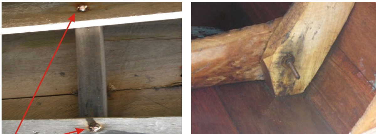
Figure 5. Bolts or Nails that Rust Easily.
